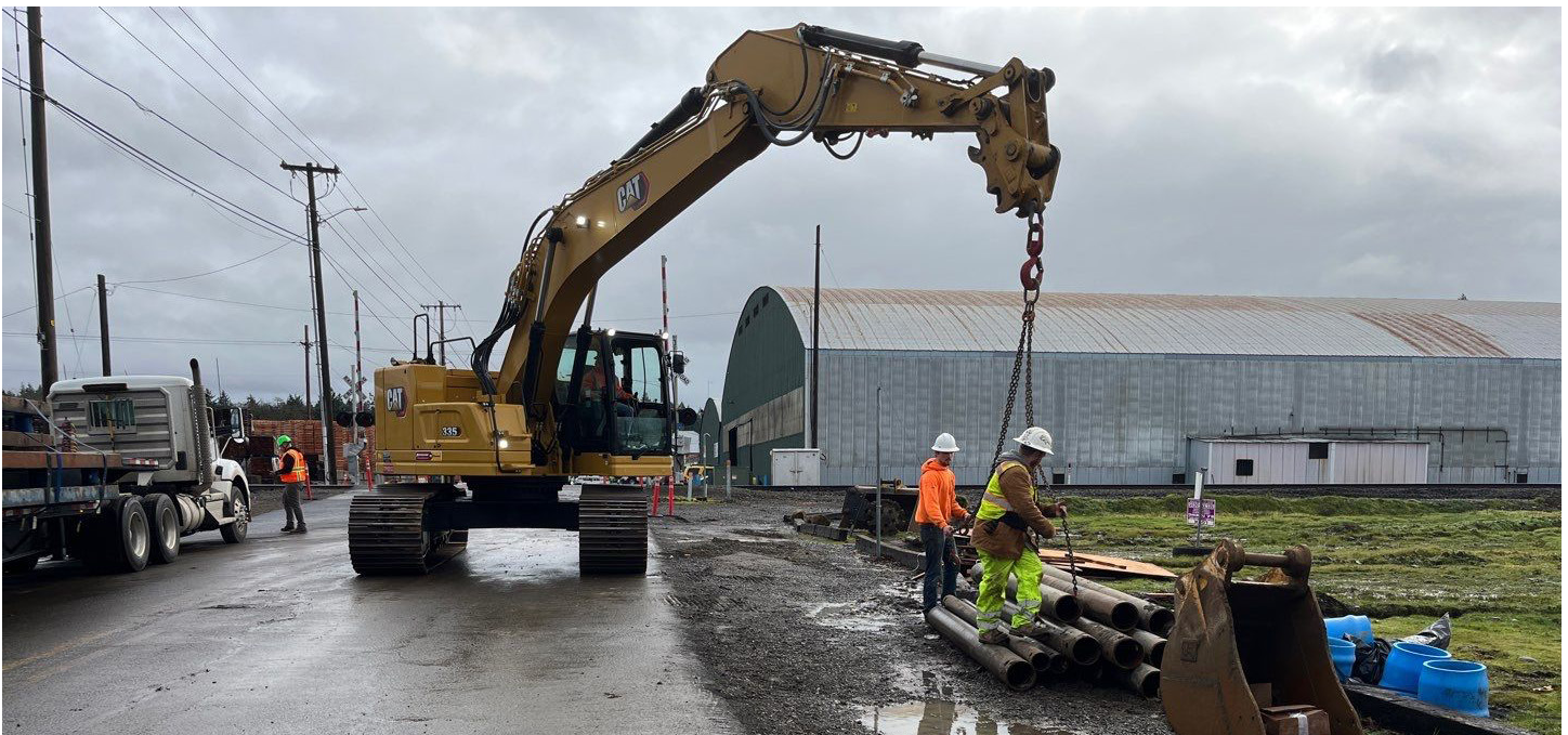
City of Turner Distribution Main
